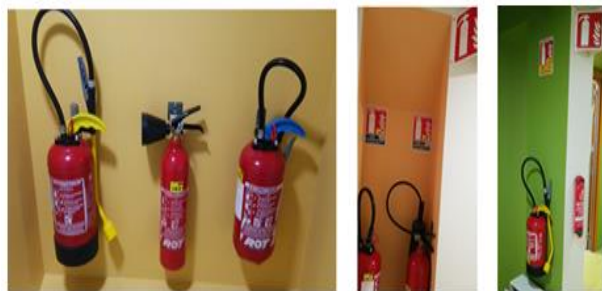
Figure 2: Fire extinguishers of a French university.
